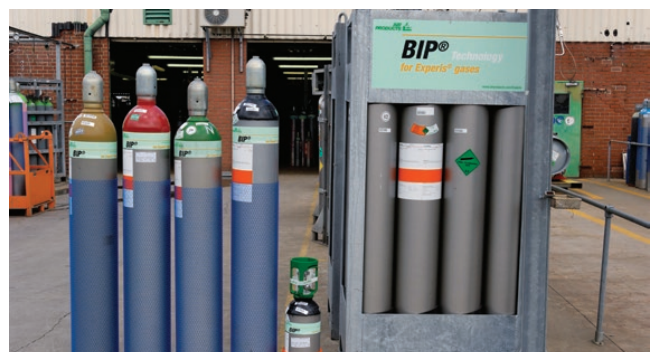
A suitable size whatever the gas requirement
